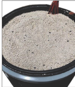
2 Loose Obexion FR poured over batteries
