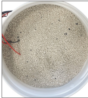
2 Loose Obexion FR poured over battery
